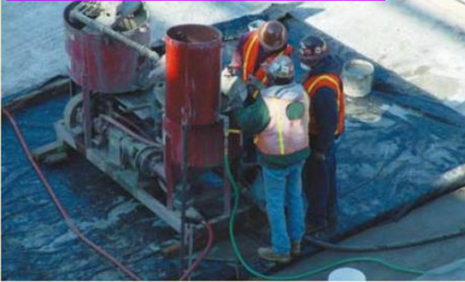
Mixing and pumping equipment
